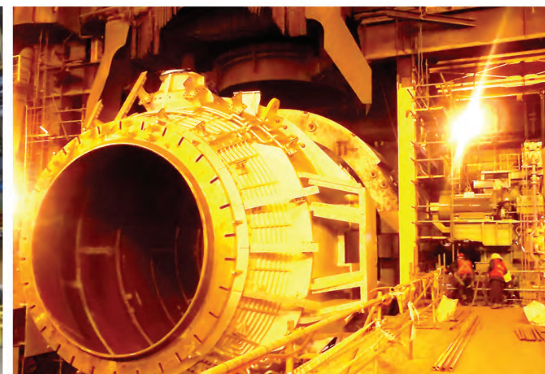
Supply of converter to the Pohang Iron & Steel Mill and Gwangyang Iron Mill
