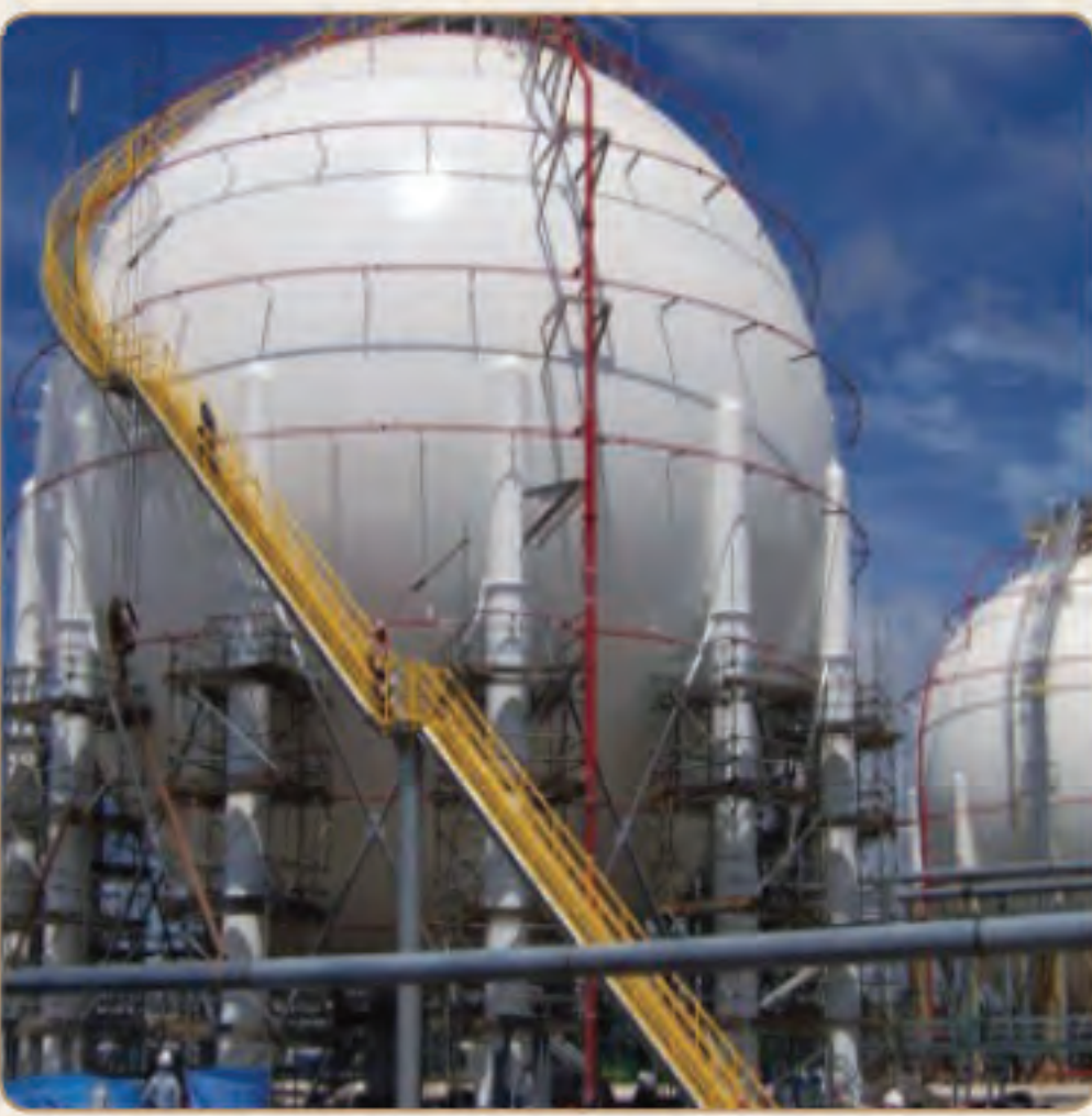
Chemical storage Tank
